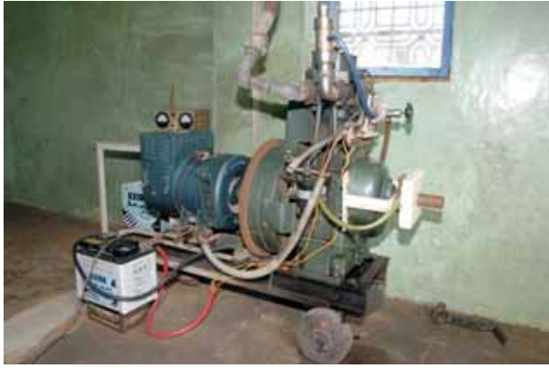
Biogas generator which operates only on gas with spark ignition
